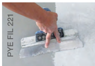
Smoothen internal surface with top coat. 第二层用抹子拉平使墙面便顺滑。
